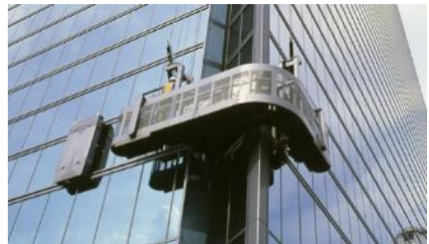
Fig. 1. Building maintenance unit [3].
