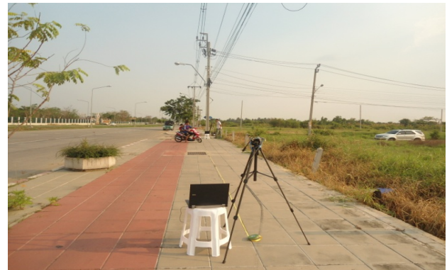
Fig. 4. Test setup for scenario 3-ZigBee meters are installed on electric power poles along an 8-lane public main road outside the community.
